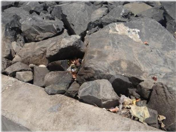
Photo 5. Accumulation of solid waste in between the openings of the basalt rocks in the dike's shell.
