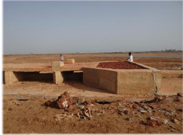
Photo 16. Scouring at the base of the rainwater discharge point and a crack in the wall.
