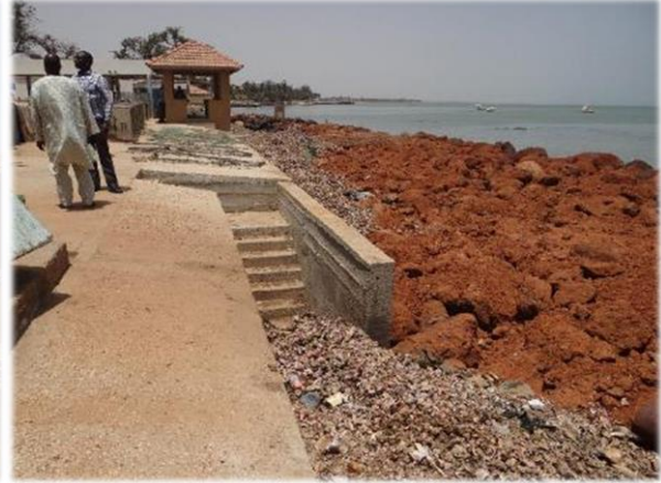
Photo 11. The basement of the fishing dock and a retaining wall rehabilitated and the replenishment of laterites financed by the AF.
