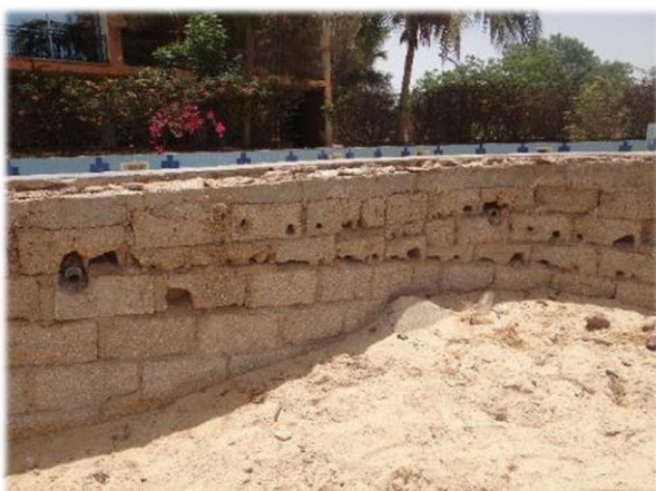
Photo 1. A pool that had been previously degraded by wave action recorded on the construction site for the seawall.
