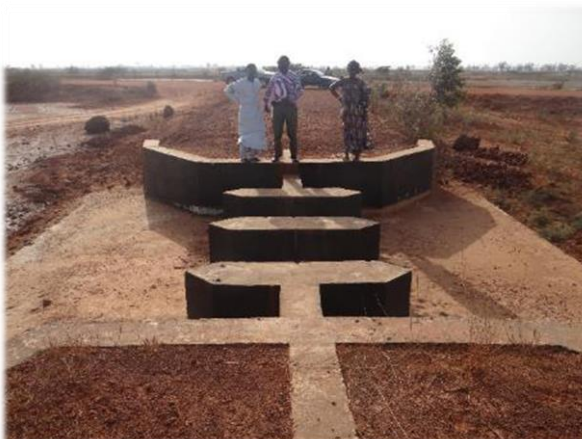
Photo 4. An element of the anti-salt dike, i.e. a rainwater discharge point, made of concrete which allows the drainage of surplus rainwater.
