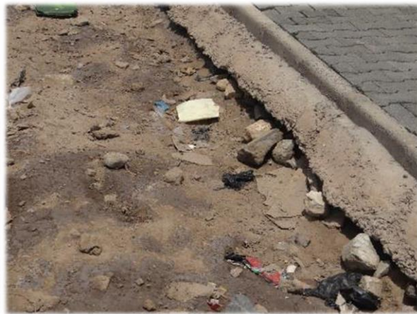
Photo 8. Scouring observed at the base of the promenade on the esplanade due to stagnant water.
